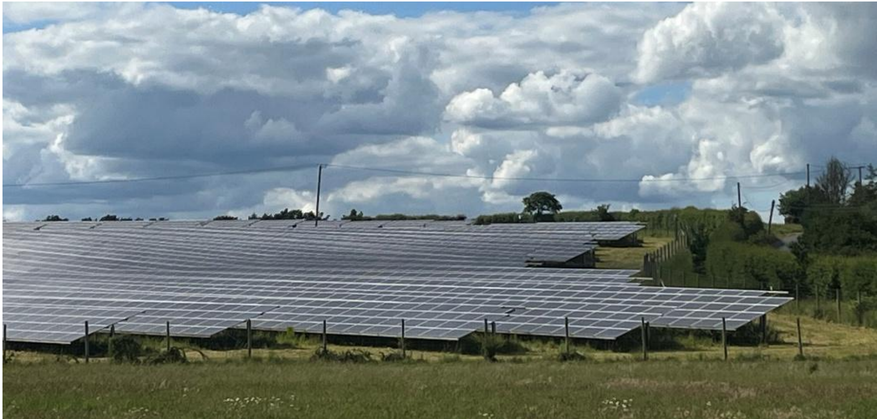
Figure 1 Example of solar panel arrays © Places Services, ECC
